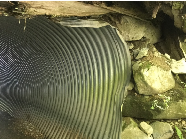
Damage at inlet
