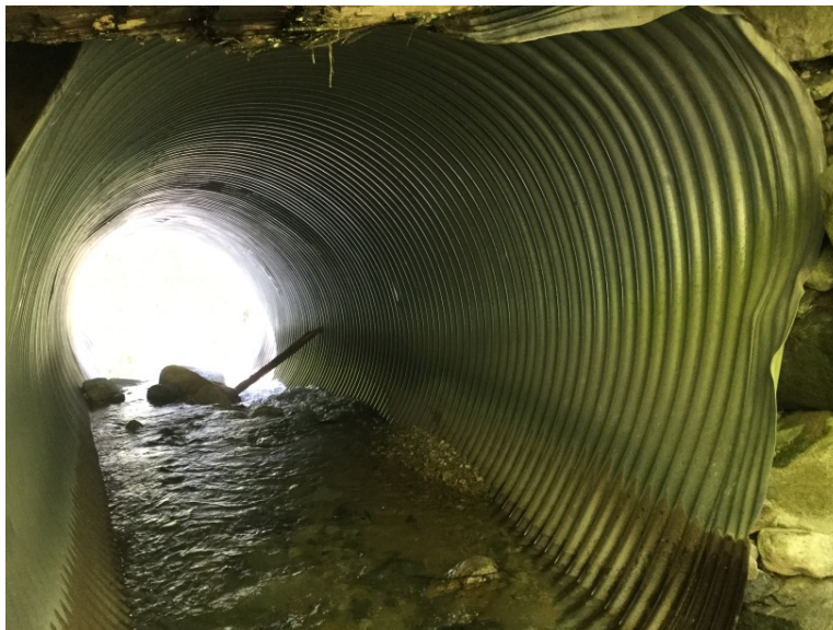
Culvert shape is not round
