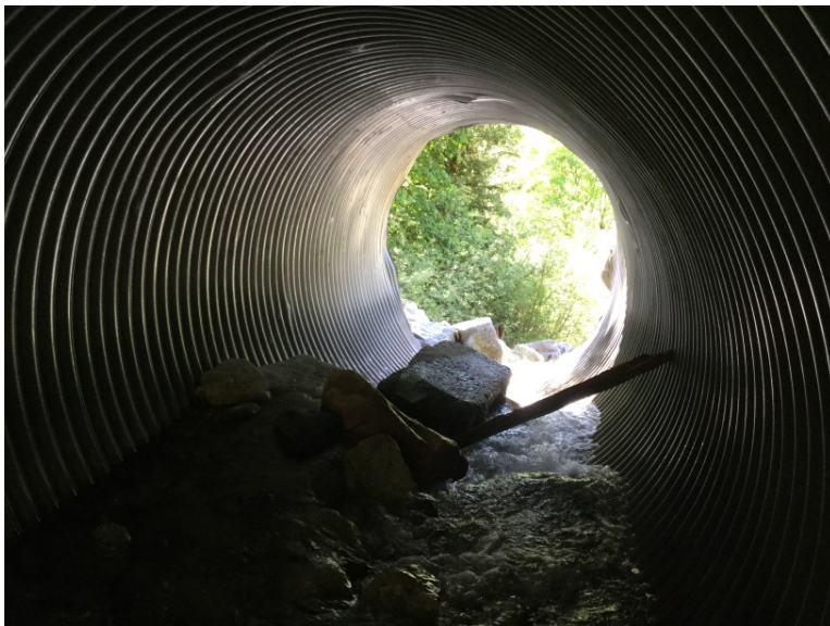
Culvert appears to have settled at outlet
